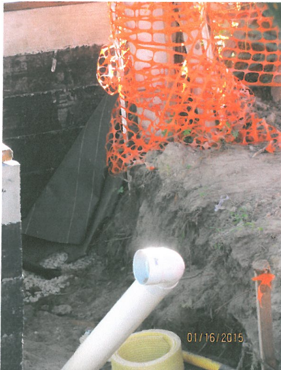
Figure No. 2. Lack of rooting soil at north side of
